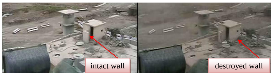
19. figure: Crash-down of a little wall due to blast effects
